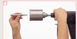
4 Only the center pin is required for positioning. Once complete positioning is made by drilling to a depth of approximately 5 mm, pull out the center pin and continue drilling operation.
